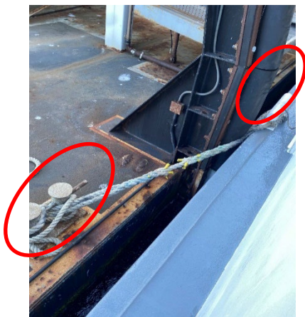
Crew stood sideways on this outboard gunwale to handle the aft spring line. The cleat was hard to access and outboard of the railing. The hook used is also pictured.
